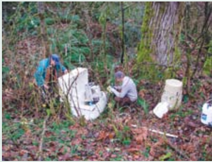
King County staff members install a flow meter and auto sampler at the tributary to Little Beaver Lake
