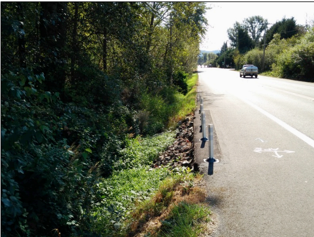
Figure 18. View of the Zackuse Creek culvert on the eastern margin of East Lake Sammamish Parkway; view is to the south.
