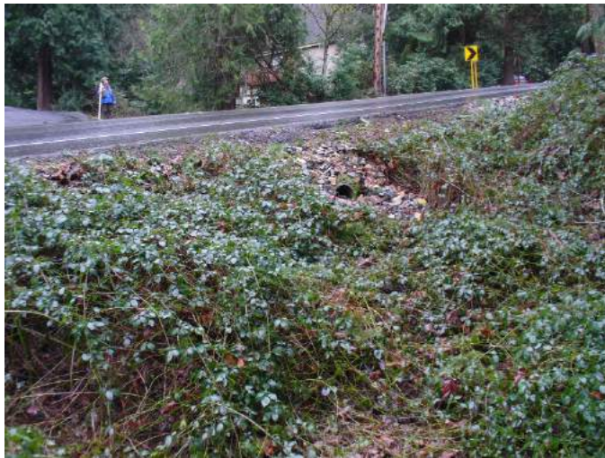
Site location: Looking north (upstream at same culvert in Photo Up-13- Outfall 1) Photo number: Up-14 Description: Looking North
