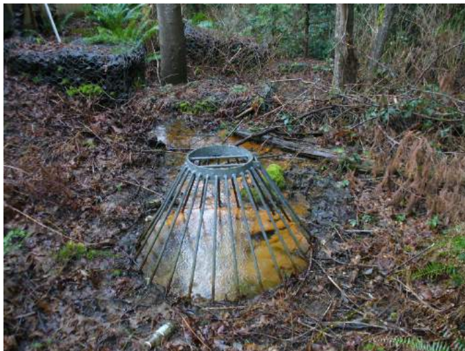
Site location: ~ 1100' upstream of birdcage east of 206 th Ave NE Photo number: Z-56 Description: Closer view of same location as Photo Z-55.
