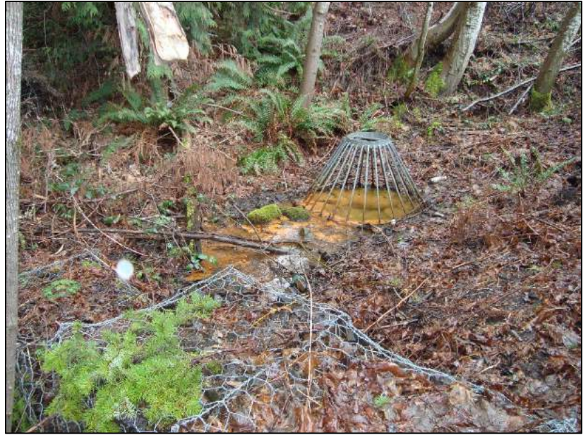
Photo 5-9. South tributary headwaters, looking upstream from first row of gabions. Orange scum on water surface is the result of oxidation. March 8, 2018.
