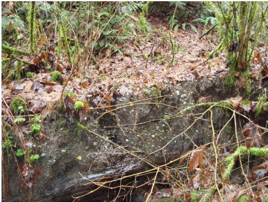
Site location: ~100' upstream of gully mouth with Zackuse Creek Photo number: Z-28 Description: Looking east at exposed sidewall of gully incised approximately 6 - 10 feet into hillslope.
