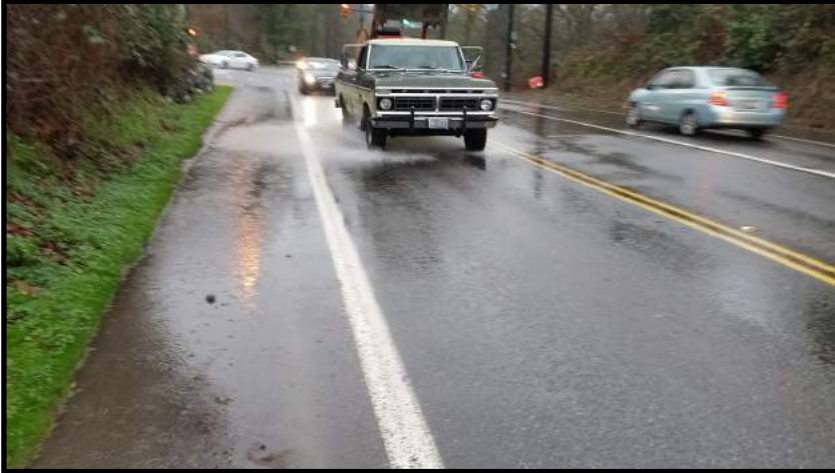
Pooling water on ELSP from seepage emanating from bank on left side of photo
