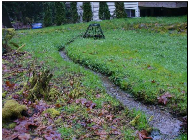
Photo 5- 11. 206th Avenue birdcage structure at the south tributary open channel terminus. 18-inch pipe is buried (see Figure 5-8 for diagram of facility at time of construction). Photo looking to the northwest. March 8, 2018.
