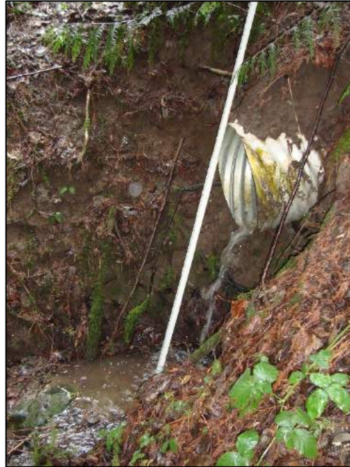
Photo 5-14. Perched culvert on private driveway south of Louis Thompson Road NE, near 210 th Avenue NE. Looking upstream toward the north. March 8, 2018.
