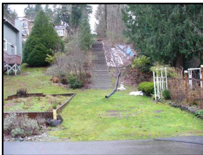
Ad-hoc stormwater drainage and failed slope (right photo)
