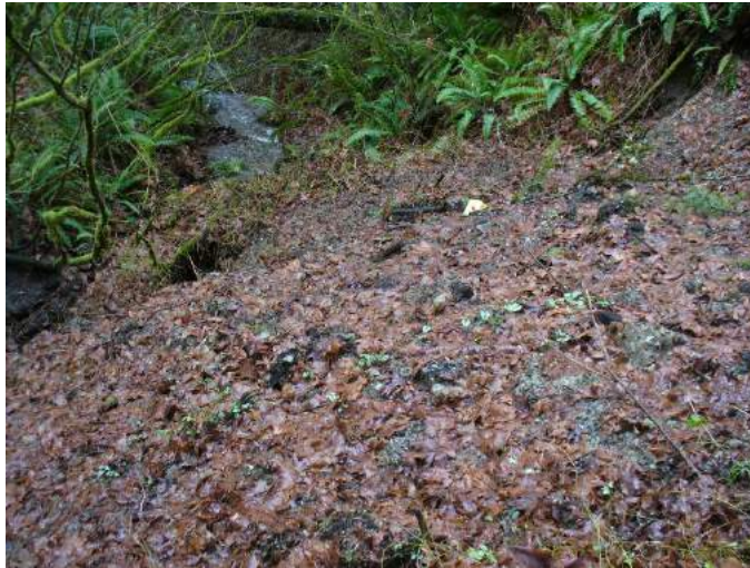
Site location: Same location as Photo Z-20 Photo number: Z-23 Description: Looking downstream direction (toward northwest), at hillslope scarp.
