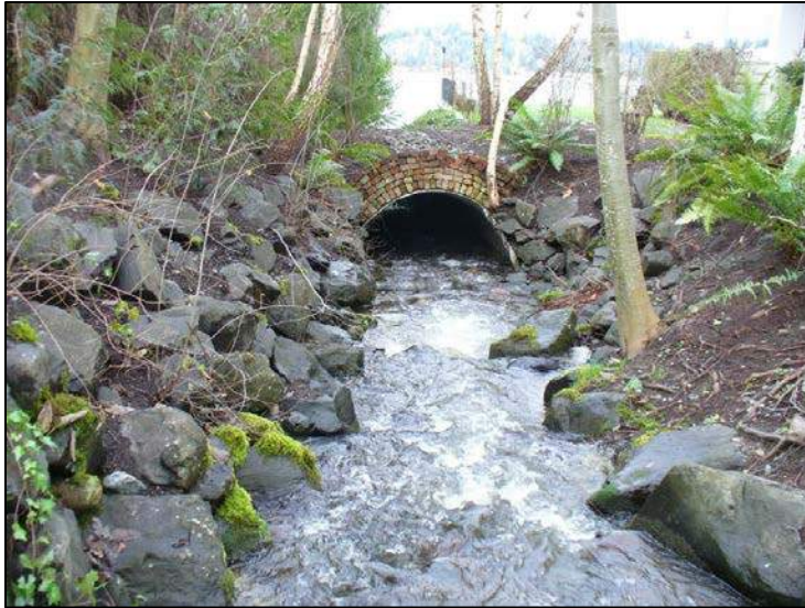
Photo 5-14. One of two 6-foot-diameter culverts along Zackuse Creek approaching the mouth. Lake Sammamish is in the background. This culvert and the other culvert (not shown) may be hindrances to fish movement but are not significant barriers. January 12, 2018.
