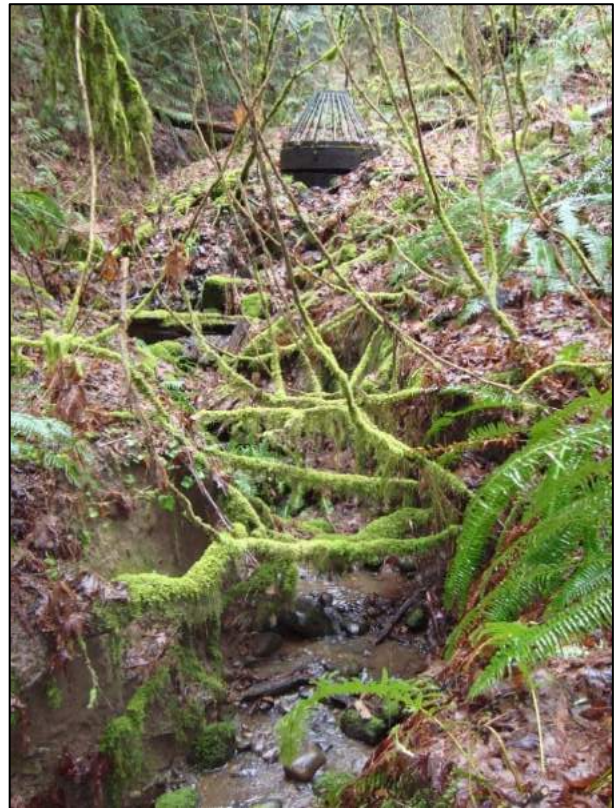
Photo 5-10. Outfall structure from West Montage vault on south tributary. Looking upstream. Erosion has occurred around outlet structure and within the channel. March 8, 2018.
