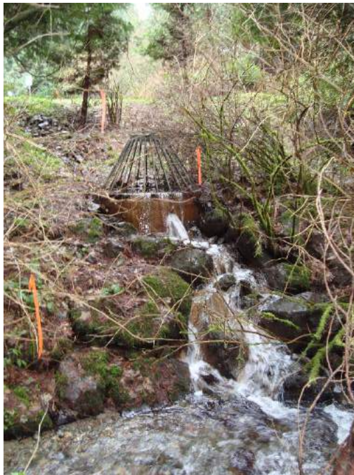
Site location: 206 th Avenue NE Photo number: Z-16 Description: Birdcage structure and energy dissipation for stormwater outfall, conveying discharge from Montage neighborhood
