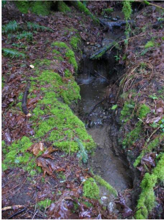
Site location: 100' upstream of birdcage near 206 th Ave NE Photo number: Z-45 Description: Incised channel through deposited sediment.
