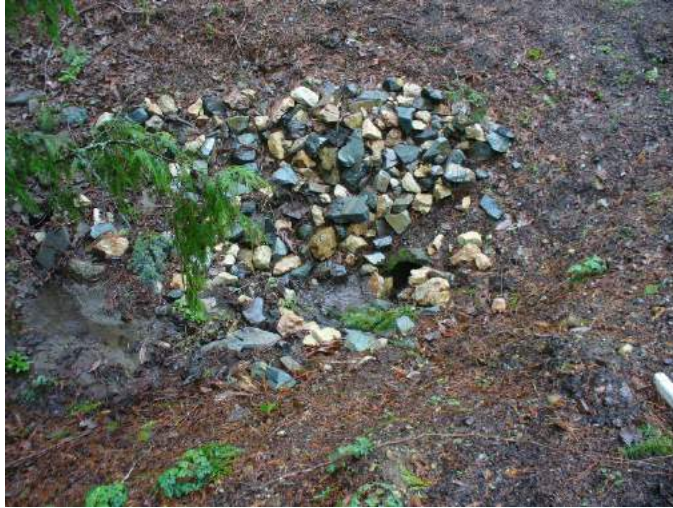
Site location: Culvert on north side of Louis Thompson Road west of 210 th Ave NE Photo number: Up-13 Description: Looking south at culvert
