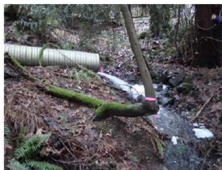
Beginning of Zackuse Creek open channel at Louis Thompson Rd. culvert
