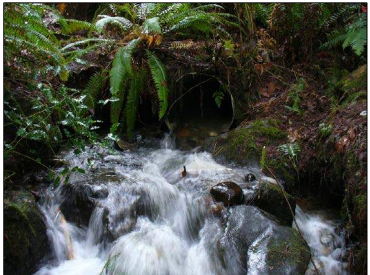
Photo 5-15. Twin 24-inch-diameter CMP culverts at 206 th Avenue NE are considered a partial fish passage barrier. Photo is looking upstream toward the east. January 12, 2018.
