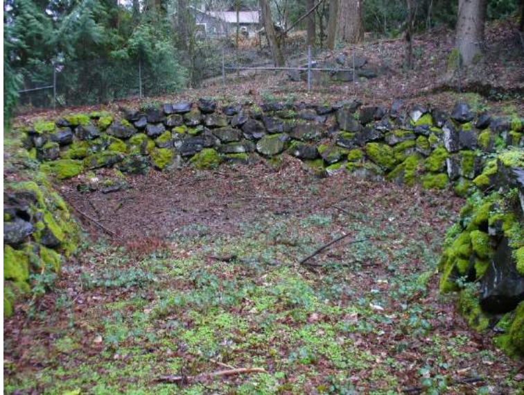
Site location: Infiltration facility (D93083) on corner of Louis Thompson Rd. and 205 th Ave NE Photo number: Up-7 Description: Looking north from Louis Thompson Rd. Pond is dry and shows no evidence of water.
