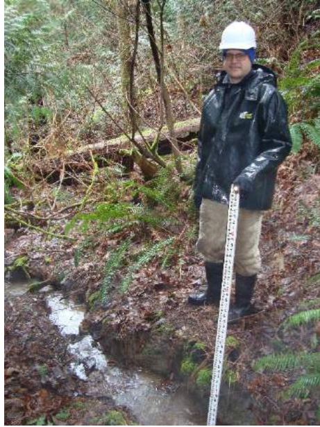
Site location: ~1000' upstream of birdcage east of 206 th Ave NE Photo number: Z-53 Description: Looking downstream at channel where incision is beginning.
